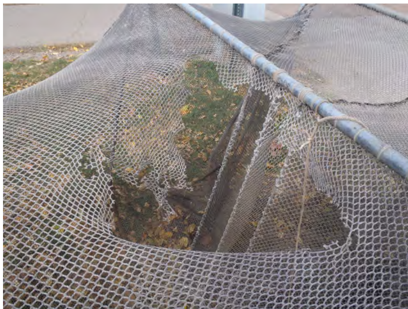
Figure 3. Net damage from Bass Lake. Results from this net were not included in the statistics.
