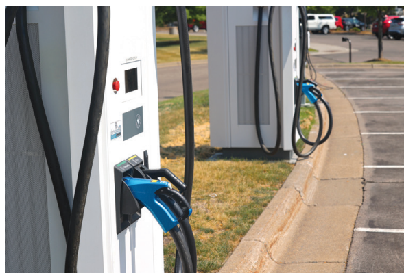
Through a partnership with CSG, the City of Plymouth offers 115 EV charging stalls across 13 locations in Plymouth.
