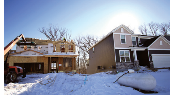
Last year, 354 single-family homes were constructed in the City of Plymouth – the highest number since 1994.
