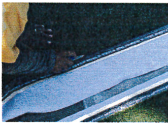
TRIM EDGES OF THE STRATUM AND SEAM W/ PB TAPE AND PB- ADHESIVE TO CREATE A FREE FLOATING PAVEMENT
