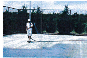
SATURATE THE INFILLED STRATUM WITH A POLYMER RESIN TO BIND ALL COMPONENTS TOGETHER
